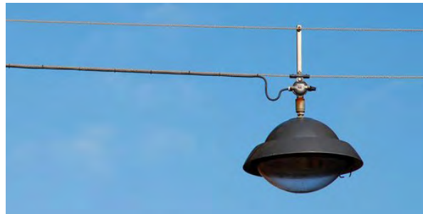
Figure 4: Catenary street lighting
