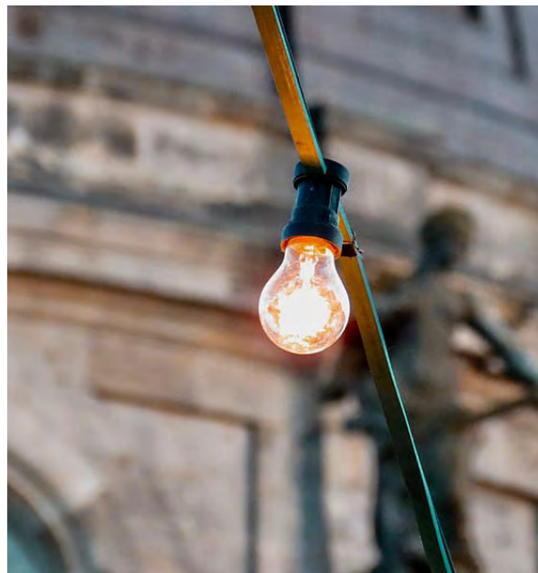
Figure 5: Catenary street lighting
